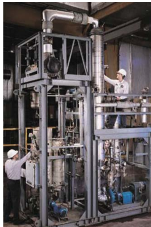
Fig. 7: Veolia's pilot scale forced ventilation evaporator.
