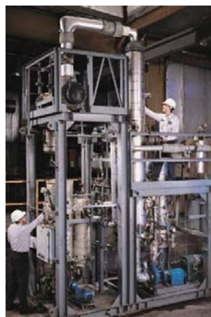
Fig. 7: Veolia's pilot scale forced ventilation evaporator.
