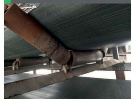
Fig 2: A corroded metal roller
