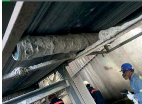
Fig 3: A return metal roller with material build-up
