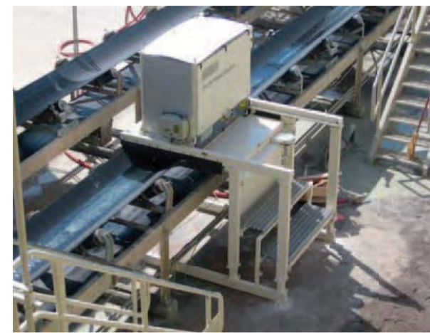
Online LIBS Analyzer Installed on a moving belt.
