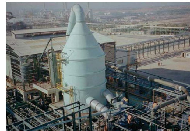
The IMACID facility at Jorf Lasfar, Morocco. OCP uses a process developed by Prayon to remove impurities from phosphoric acid.
