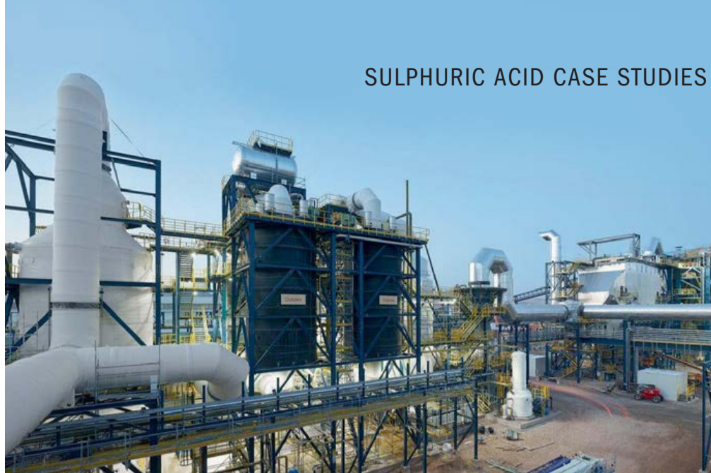
Mazidagi's gas cleaning plant section.
