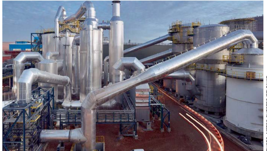
Mazidagi's sulphuric acid plant.
