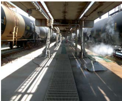
Steam feeds to liquid sulphur rail cars.
