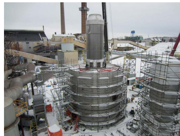
Fig. 4: Chemetics stainless steel converter with internal exchanger.
