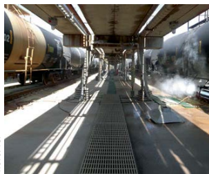
Steam feeds to liquid sulphur rail cars.
