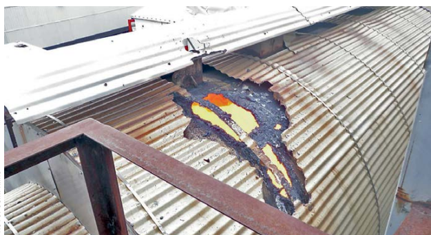
Fig.4: Result of overheating of the main combustion chamber.
