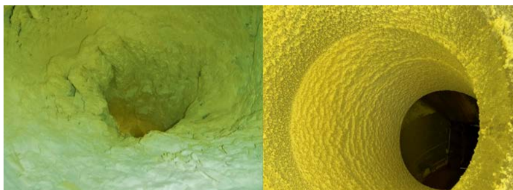
Fig. 2: Major build-up (left) vs. minor build-up (right) inside ducting.
