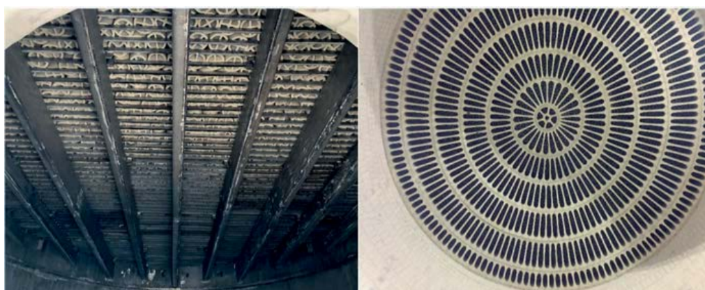
Fig. 2: Acid tower packing support. Project A (left): metallic support. Project B (right): self-supported ceramic dome.
