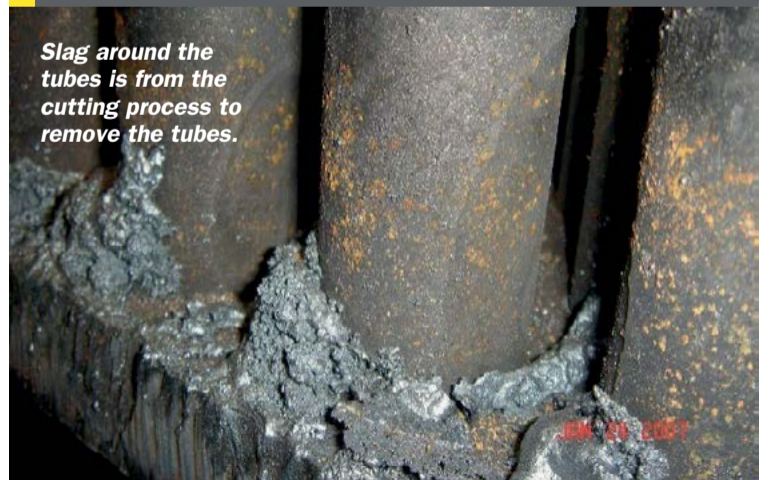
Fig. 10: FAC corrosion on bottom of tubes at the hot gas inlet
