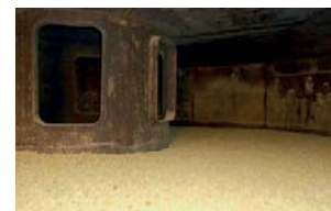
Fig. 3: Reactor bed of Quattro catalyst.
