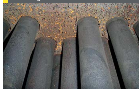
Fig. 15: Condenser inlet tubes – dissolved oxygen pitting during shutdown
