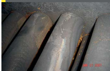
Fig. 14: Last condenser – corrosion on bottom of tubes at the hot tubesheet
