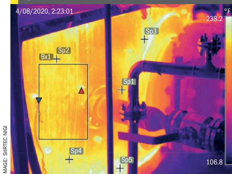
Fig. 8: WHB rear channel skin temperature measurement
