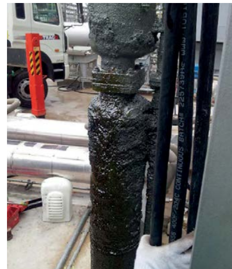
Fig. 12: CarSul on sulphur pump.
