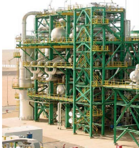
TGTU re-start at Mellitah complex, Mar/Apr p38.
