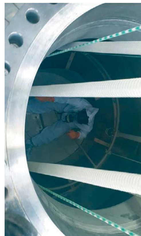
Fig. 3: Loading of tertiary catalyst.
