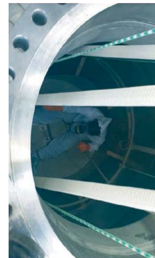
Fig. 3: Loading of tertiary catalyst.
