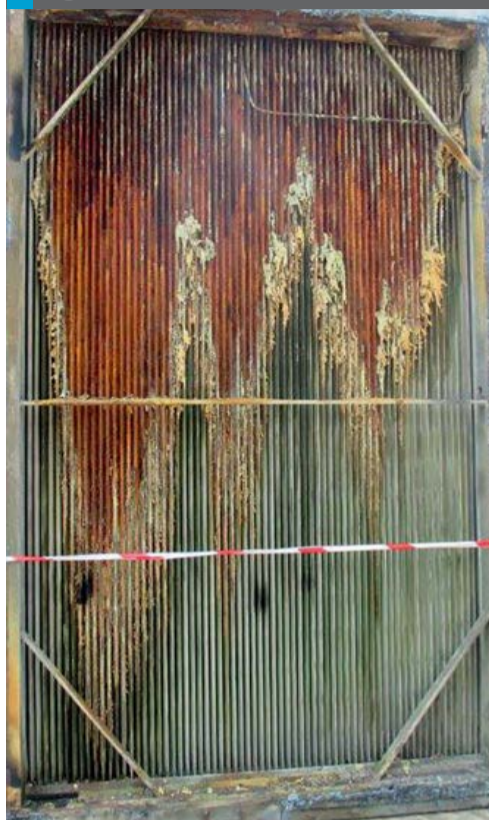
Fig. 1: Corroded metallic APH
