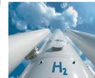
Hydrogen tanks at a Linde facility.
