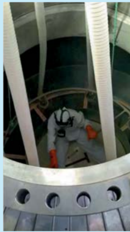
Fig. 6: Remote assisted commissioning of reactor catalyst
