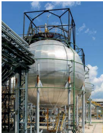
Cover: Ammonium storage tank at a refinery. Bolbik/Shutterstock.com
