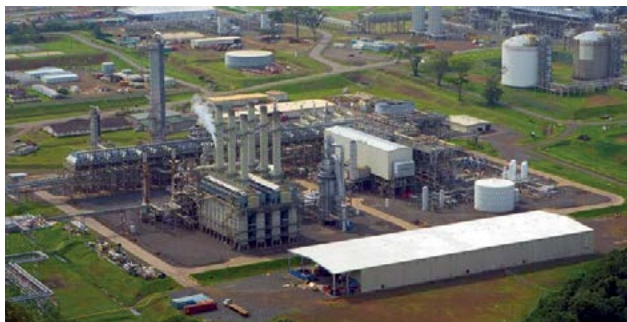
The Atlantic Methanol Production Company (AMPCO) methanol plant at Punta Europa, Equatorial Guinea.
