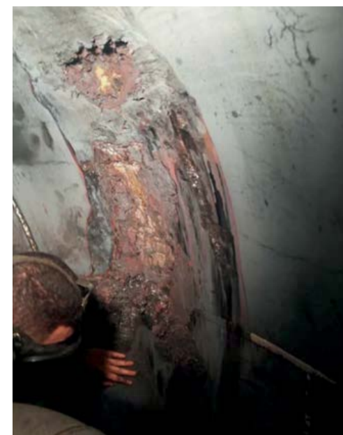
Fig. 7: Damage behind the lining of a HP scrubber.
