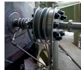
Fig. 16: Installed radar – external view with heat tracing.
