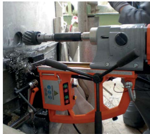
Fig. 14: Drilling of hole in existing vessel for installation of new radar nozzle.
