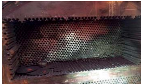
Fig. 3: CS part of tubesheet removed for weld overlay inspection.
