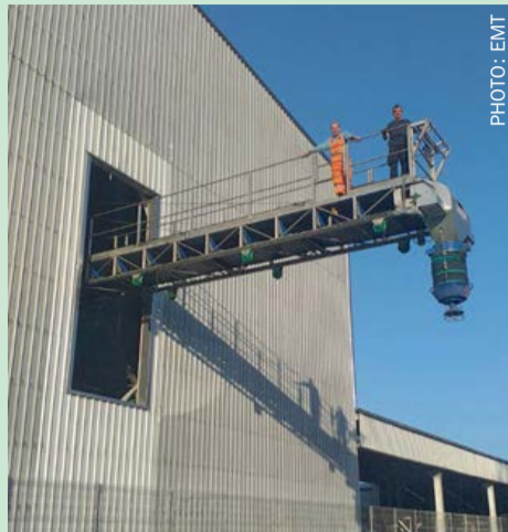
EMT train filling shuttle conveyor, ISAOSA blending plant, Topolobampo, Mexico.
