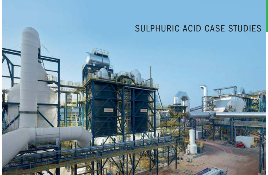
Mazidagi's gas cleaning plant section.
