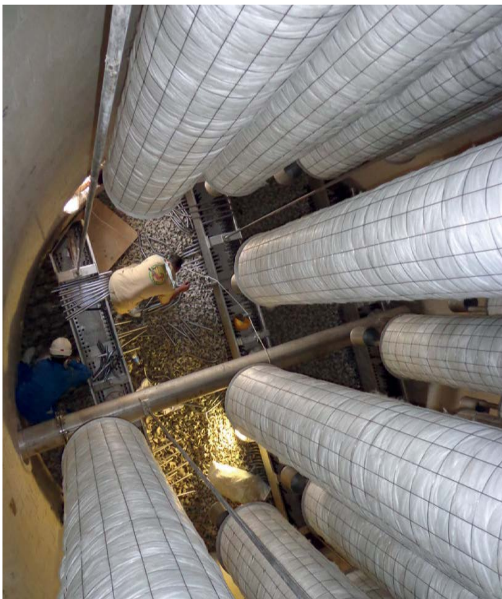
A view of the MECS® Brink® mist eliminators in the new acid tower.
