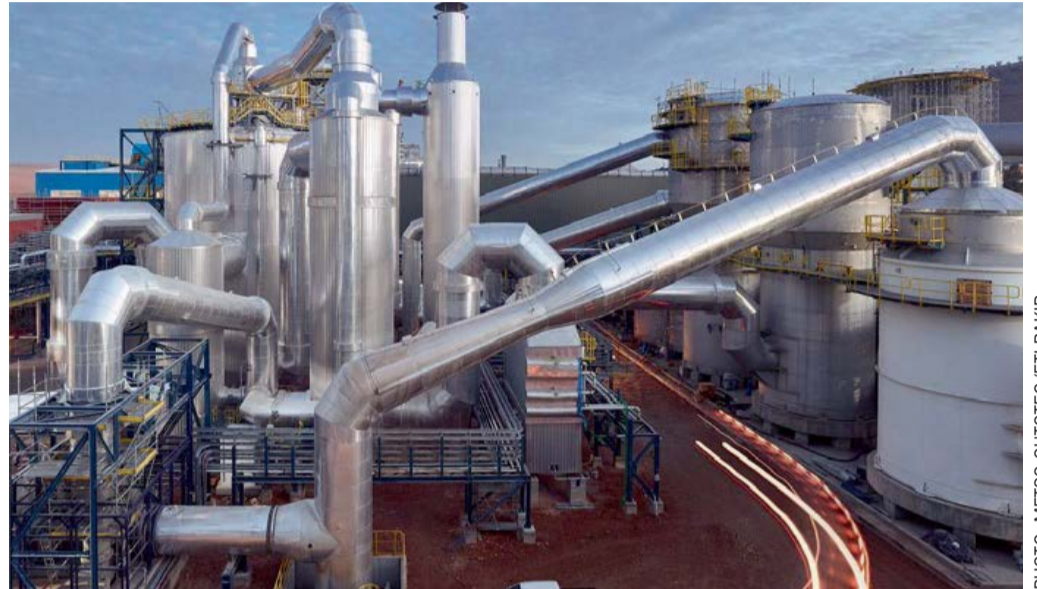
Mazidagi's sulphuric acid plant.
