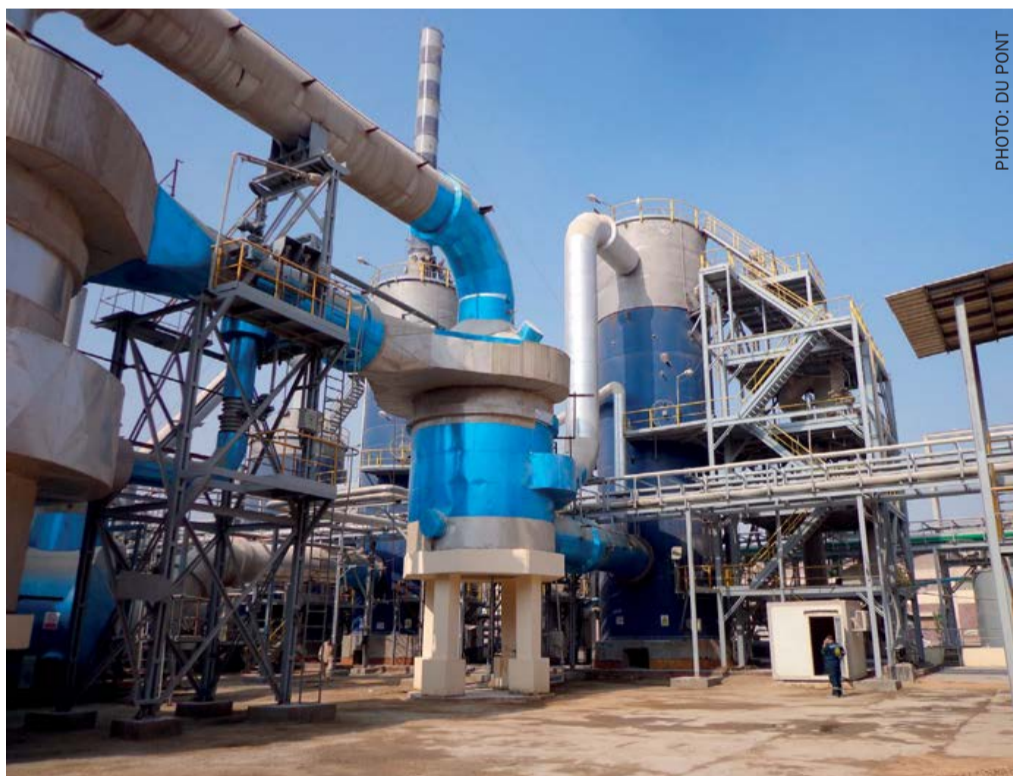
AZFC's Unit 6 after the revamp project.
