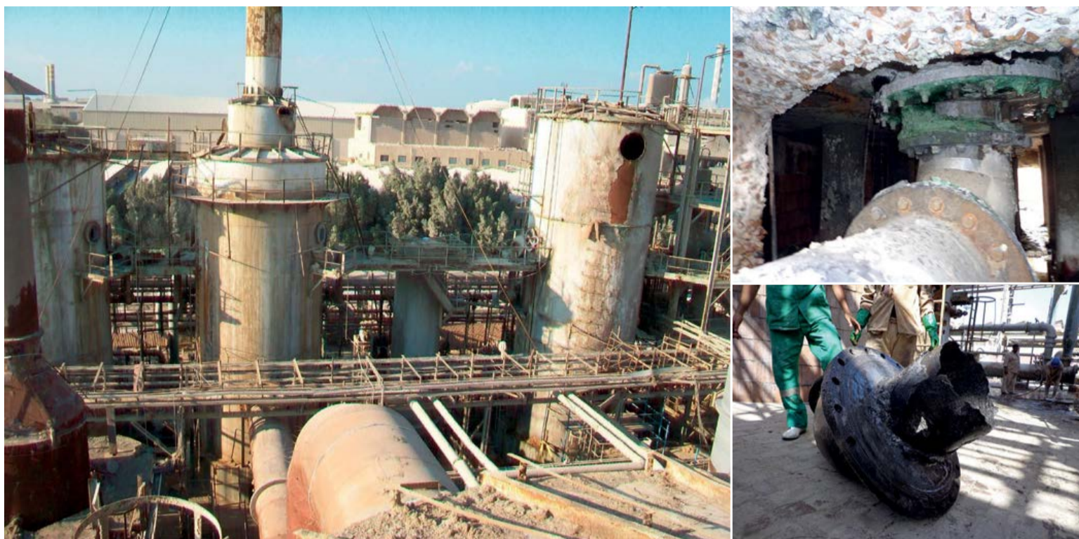
Above left: AZFC's Unit 6 before the revamp– the drying and absorption towers were in very bad shape. Above right (top and bottom): Acid was leaking from the bottom of the acid tower, causing corrosion issues.
