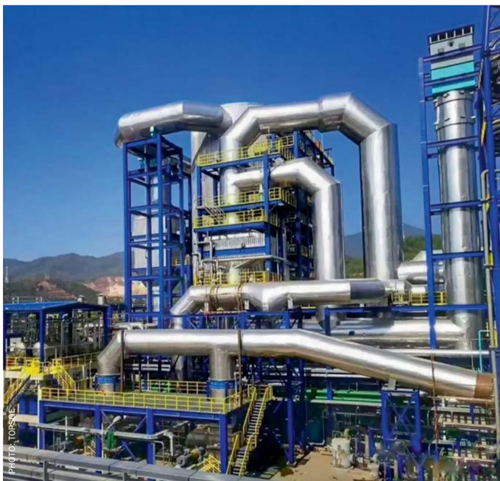
A Topsoe WSA plant at Bestgrand Chemical Group, Guangdong, China. The plant processes spent acid from the neighbouring CNOOC refinery.
