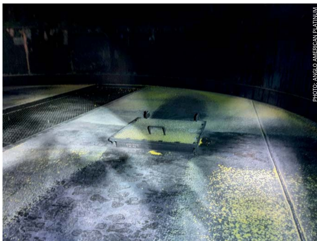
Fig. 5: Inspection showing the hatch with only 2 out of 16 bolts, and clear pattern of gas having passed through.
