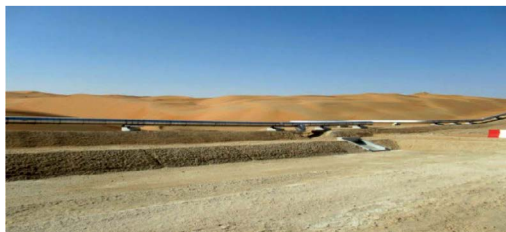
Fig. 7: Drain and drain pit for the new sulphur pipeline; 1 m elevation increase to avoid sand accumulation.
