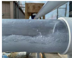
Example of liquid turbulence exiting the vertical drop.
