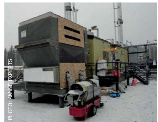
Fig. 9: Creative solution for a missing section of the amine cooler and reflux condenser.
