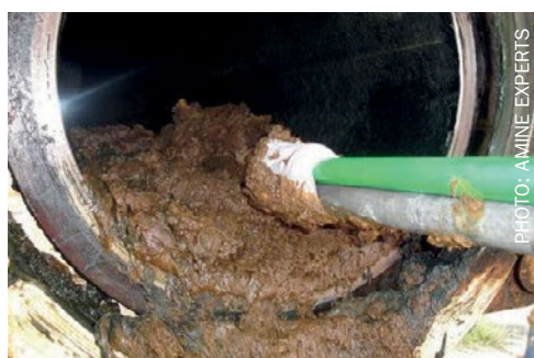
Fig. 2: Waxy solids removed from inlet slug catcher.
