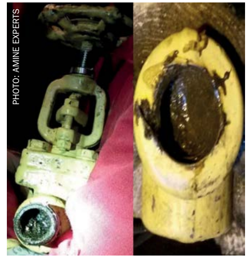
Fig. 7: Valves plugged with silt and unit full of potential fouling and foaming material.
