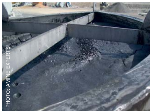
Fig. 4: Fouled activated carbon bed.
