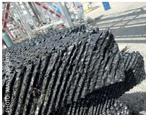
Fig. 3: Fouled flash drum coalescer pads.
