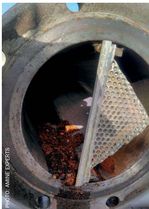
Fig. 12. Debris found during flushing.
