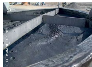
Fig. 4: Fouled activated carbon bed.
