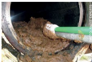
Fig. 2: Waxy solids removed from inlet slug catcher.
