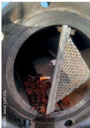
Fig. 12. Debris found during flushing.
