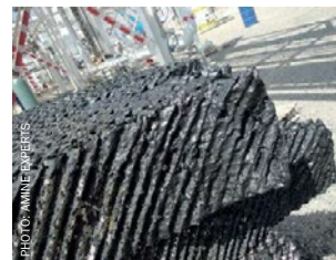
Fig. 3: Fouled flash drum coalescer pads.
