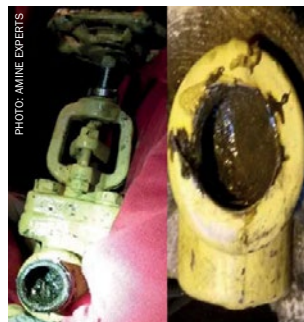
Fig. 7: Valves plugged with silt and unit full of potential fouling and foaming material.
