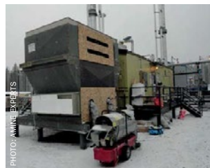
Fig. 9: Creative solution for a missing section of the amine cooler and reflux condenser.
