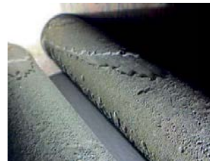
Fig. 14: Oxygen pitting on condenser tubes.
