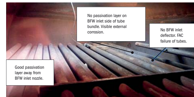
Fig. 2: Flow-accelerated corrosion caused by disturbance at the BFW Inlet
