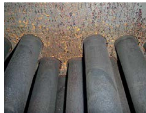
Fig. 13: Oxygen pitting on condenser inlet tubesheet.
