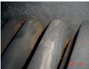
Fig. 12: Corrosion at 6 o'clock on condenser inlet tubesheet.
