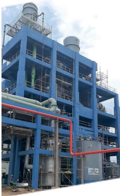
Phosphoric Acid Concentration Unit, Commissioned Oct 2021
