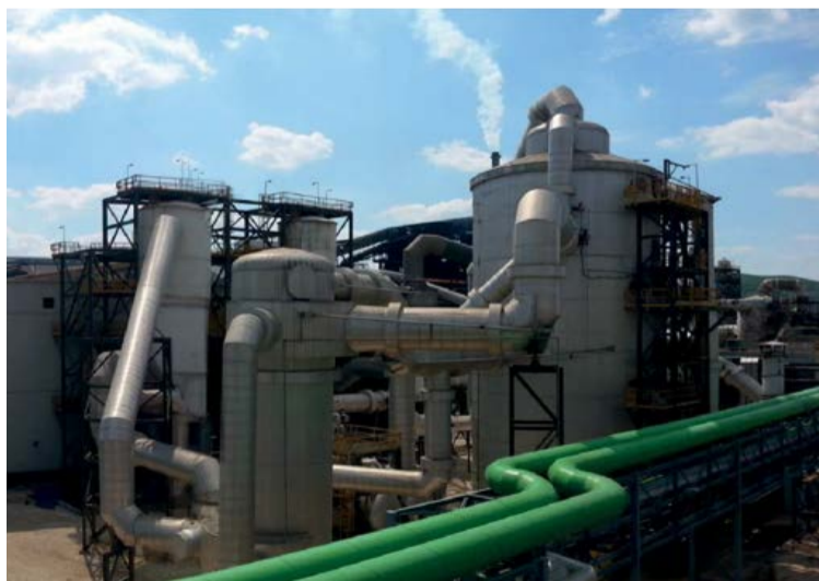
A sulphuric acid plant in a pyrometallurgical complex.
