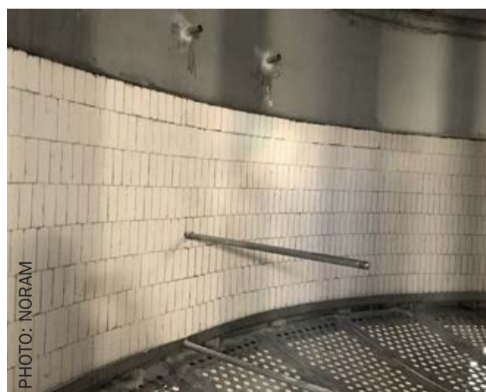
Fig. 4: Refractory lining of converter first pass.
