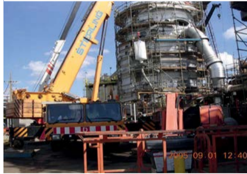
Fig. 6: Replacement converter in a new location.
