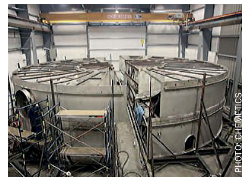
Fig. 13: Two half ring modules per level for smaller converters.
