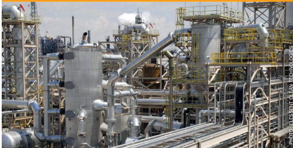
A MECS sulphuric acid plant.
