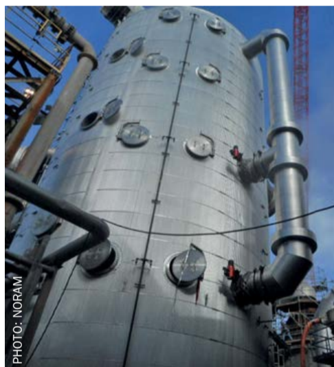
Fig. 3: Manways and start-up bypass duct.
