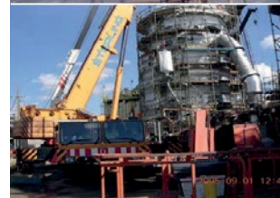
Fig. 6: Replacement converter in a new location.
