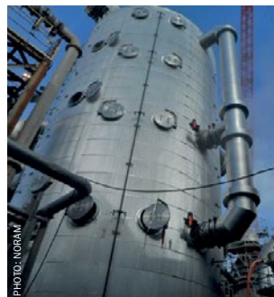
Fig. 3: Manways and start-up bypass duct.
