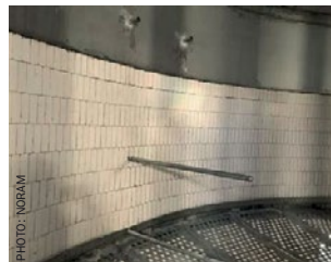
Fig. 4: Refractory lining of converter first pass.
