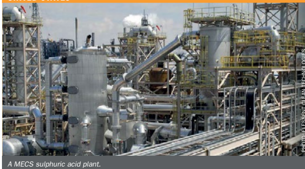
A MECS sulphuric acid plant.
