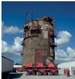
Fig. 7: Demolition and wheel out (left) and wheel in of new converter (right).
