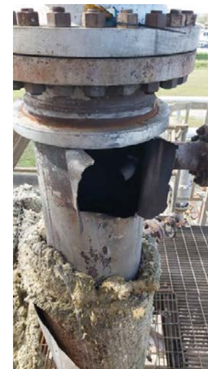
Fig. 4: Close view of the failed stripper
