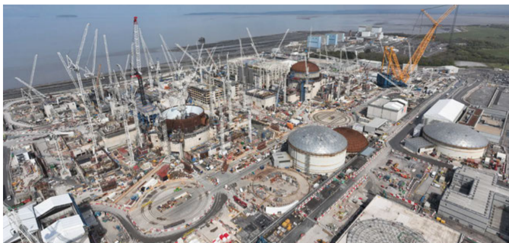
Construction of the new nuclear power plant at Hinckley Point C, UK.
