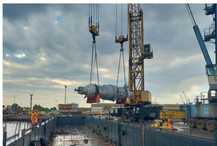
PHOTO: BELLELI ENERGY
