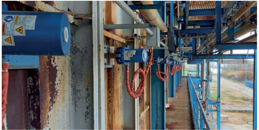
Fig. 10: Photo of installed ZoloSCAN sensor heads on the reformer at Yara Le Havre.
