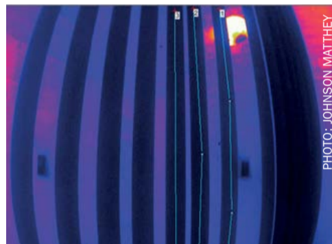
Fig. 6: Still image from video recorded by Reformer Imager, showing sections of reformer tubes.
