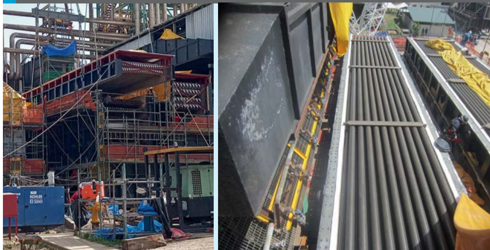
Fig. 3: New steam super heating coils (hot and cold) supplied by Casale
