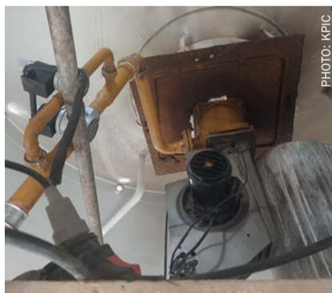
Fig. 12: View of burner and its fan in the bottom manhole.
