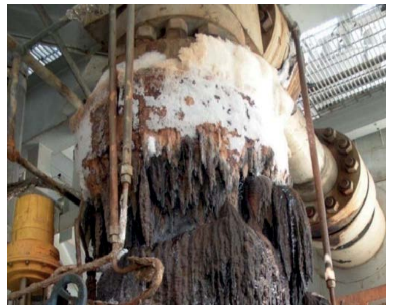
Fig. 1: Solids have stopped the leak but created a critical unsafe situation.
