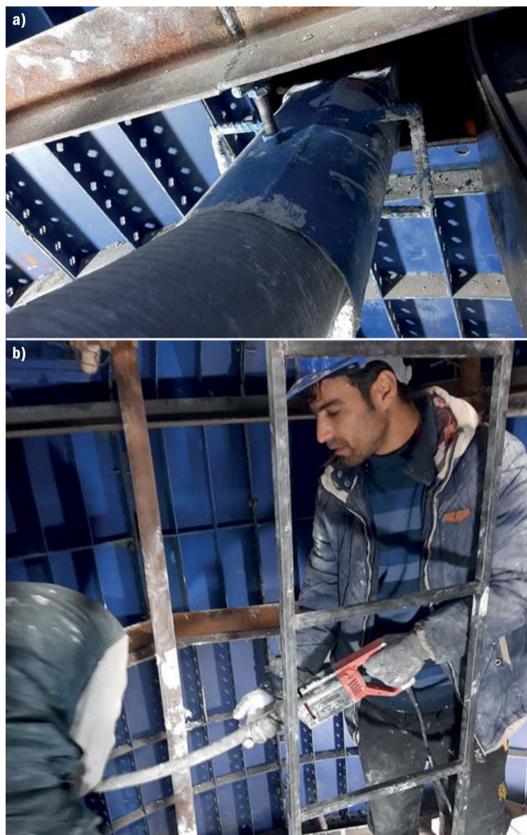
Fig. 9: a) Draining the casting material into the opening of forms through a flexible hose and chute; b) Internal vibrator via the window opening.
