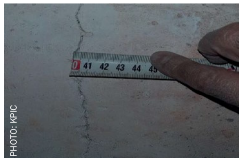
Fig. 14: Measuring the width of cracks after dryout.
