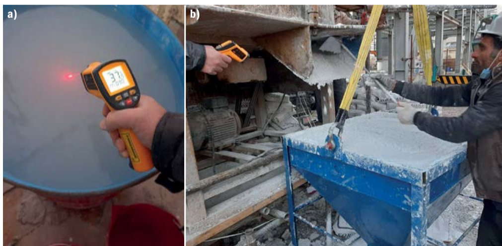
Fig. 6: a) Measuring the temperature of water; b) Pouring refractory into the hopper.
