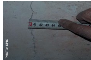
Fig. 14: Measuring the width of cracks after dryout.
