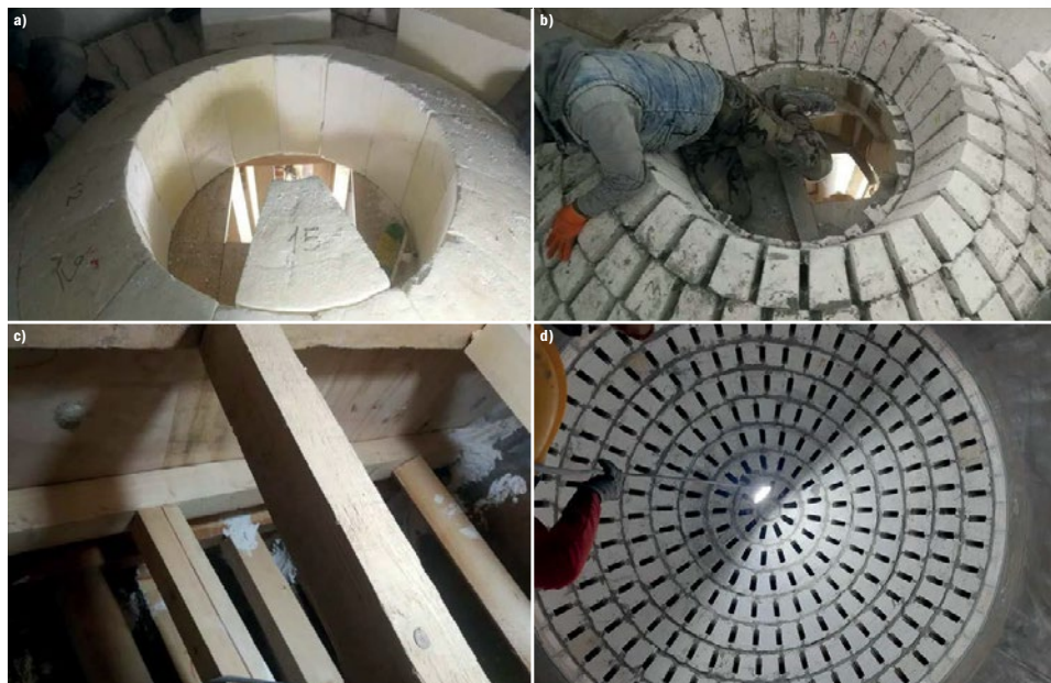
Fig. 11: a) View of polystyrene forms; b) Installation of dome bricks; c) View of wooden beams and probes; d) Final dome brick from bottom view.
