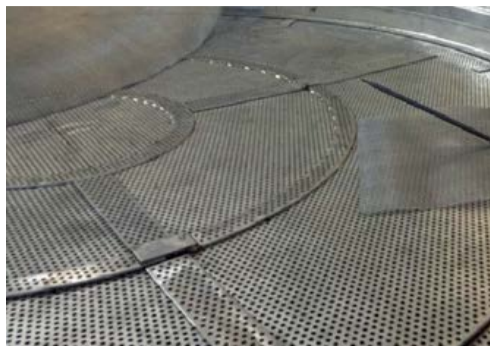
Fig. 6: Inside of a basket in good physical condition and with an even and level support.
