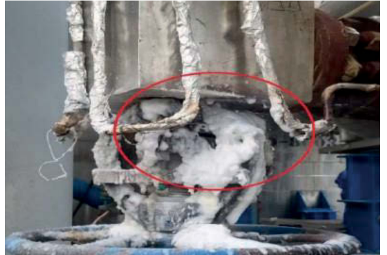
Fig. 3: Leaks along a threaded bonnet connection of a high-pressure drain valve.
