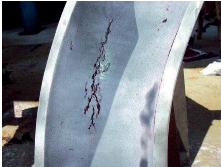
Fig. 4: Cracks in a high-pressure carbamate gas line.
