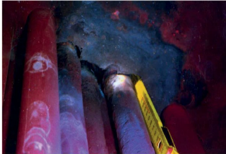
Fig. 2: Severe corrosion of the carbon steel tubesheet due to a leak in a tube.
