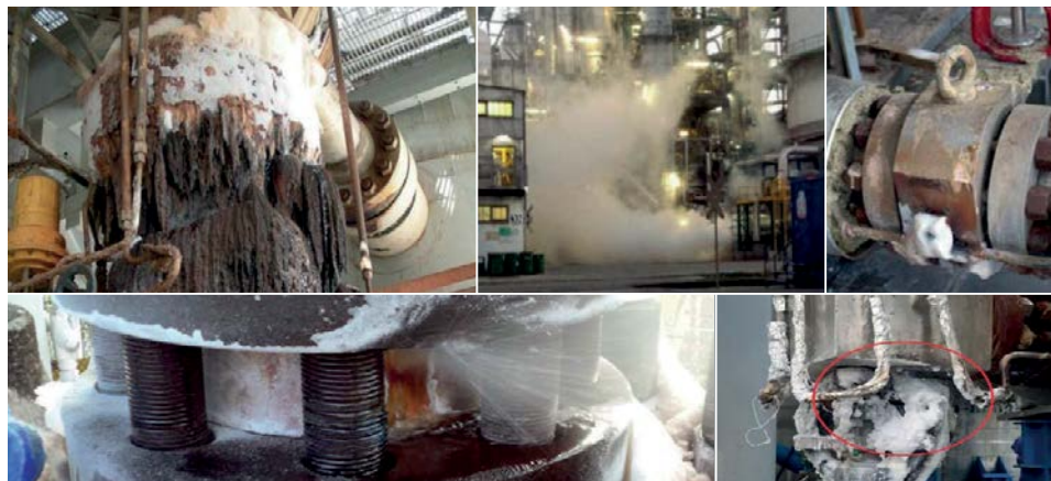
Several examples of leaks in urea plants.
