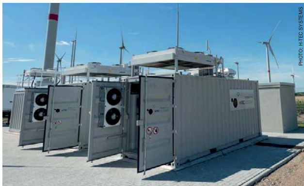
Fig. 3: PEM electrolyser by H-TEC SYSTEMS.
