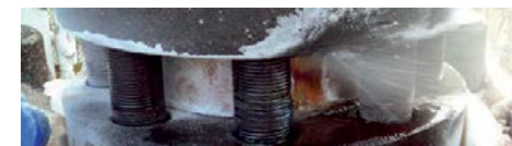
Fig. 5: A typical leak of a lens ring flange connection.
