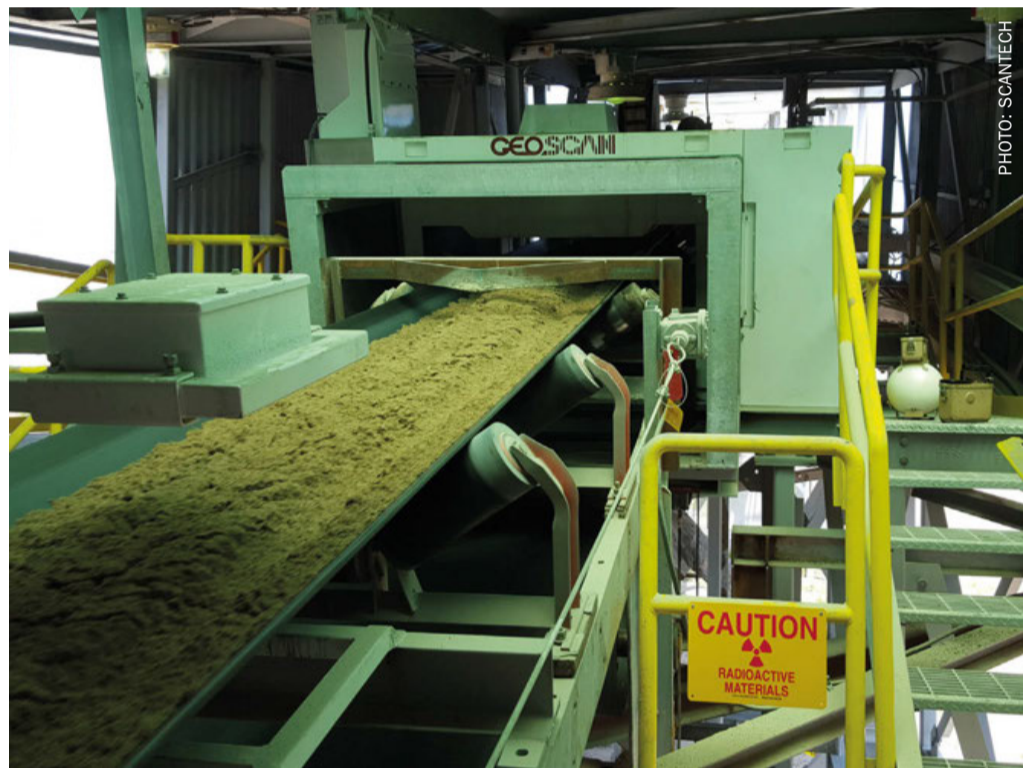
North American Geoscan-M installation for monitoring beneficiated phosphate – with a TBM moisture analyser in the foreground.
