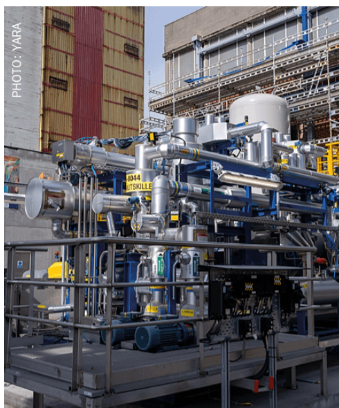
The 24MW renewable hydrogen plant at Herøya Industrial Park in Porsgrunn, Norway, is the largest of its kind currently operating in Europe.
