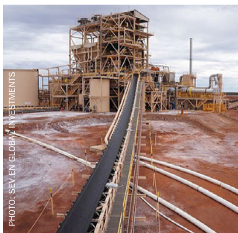
SO4 is commissioning its SOP processing plant at Lake Way, Western Australia, having made a substantial investment in the project since 2022.
