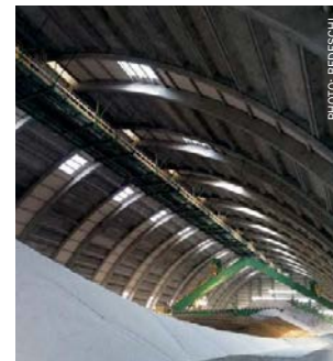
A Bedeschi 2,400 t/h fertilizer reclaimer installed at OCP's Jorf Lasfar complex in Morocco.
