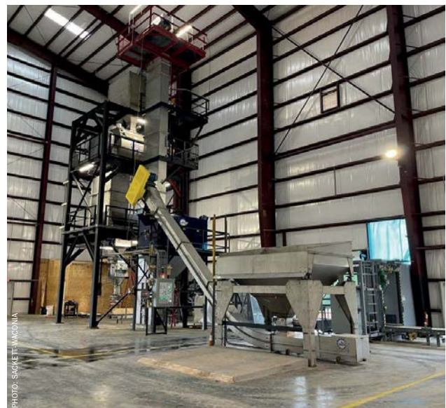
Blending/bagging system installed for Beaty Fertilizer in Cleveland, Tennessee.
