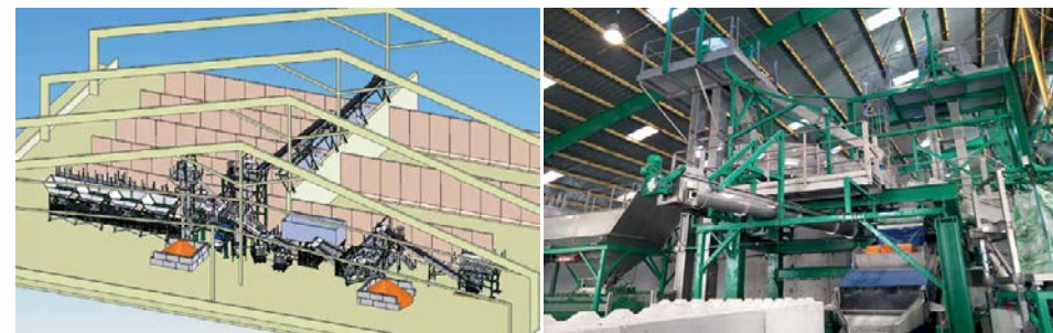
EMT successfully installed a state-of-the-art fertilizer production line for Atena at La Rochelle-Cedex, France.
