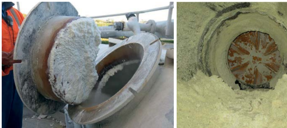
Silica deposits (left) are a natural and unavoidable by-product of scrubbing. These need to be carefully managed to avoid blocking pipes, ducts and fans (right).
