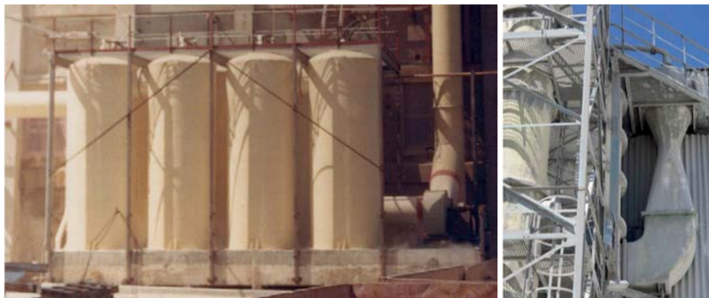
Traditional void towers (left) struggle to meet today's strict emissions limits. Venturi scrubbers (right), while a common solution, also have several limitations.
