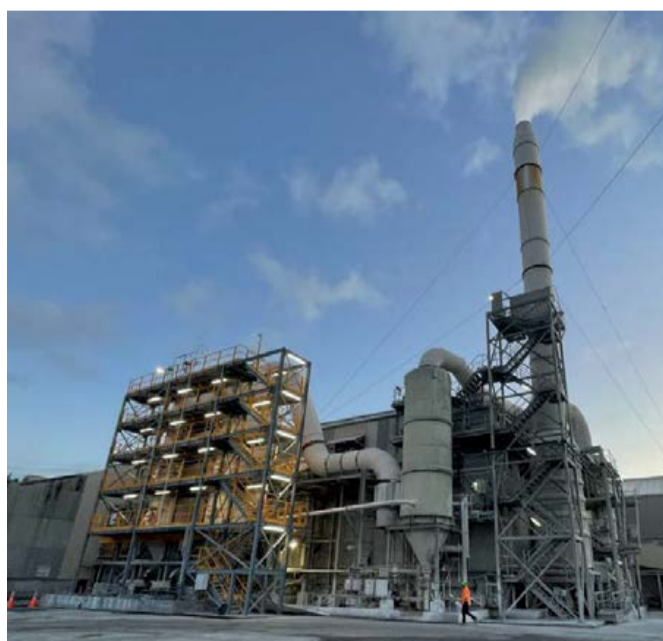
Case study 2: Phase 1 of the SSP scrubber upgrade (left) helped the client win an environmental award. The recently completed phase 2 of the upgrade (right) has future-proofed the site for increased production.
