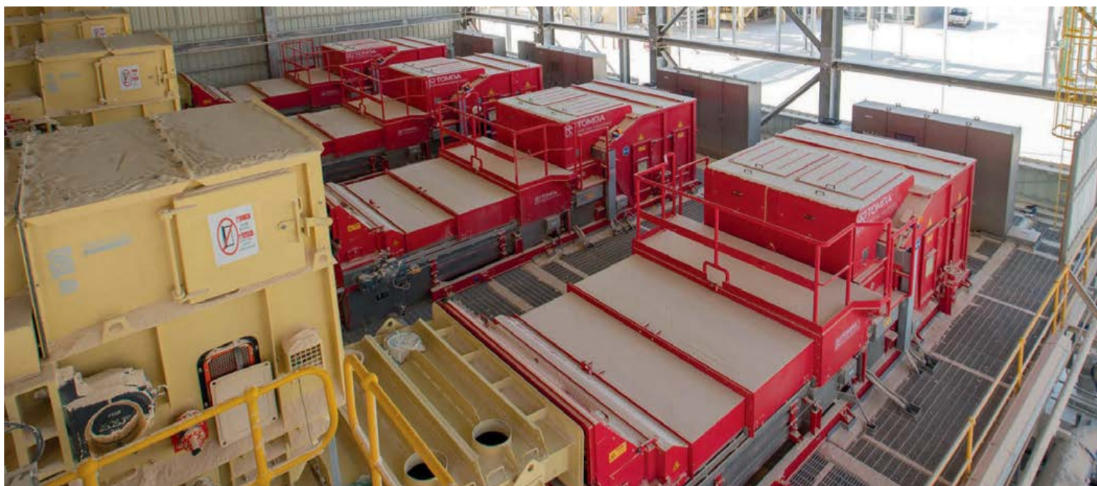
An array of four TOMRA sorting machines at the MWSPC mega project in Saudi Arabia.
