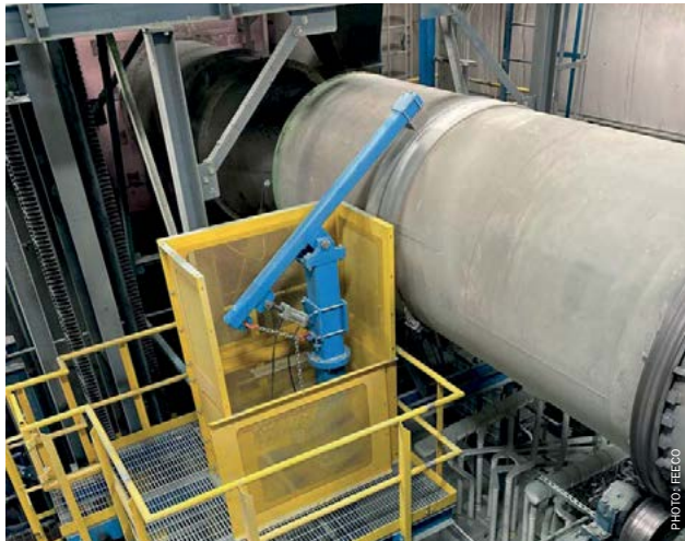
A pneumatic hammer knocker mounted on the side of a rotary dryer.
